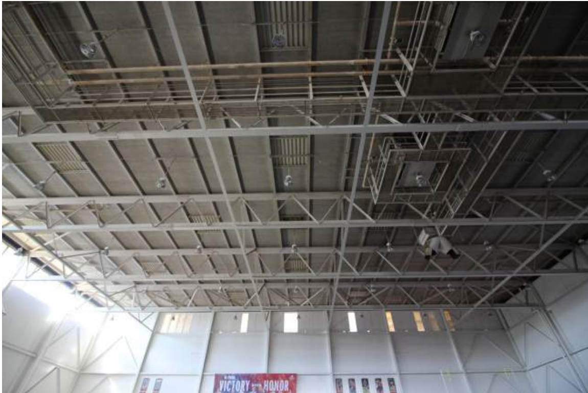
DHR Identification Number: 104-5292 June 4, 2018 Quinn Evans Architects Cage interior looking south at ceiling.
