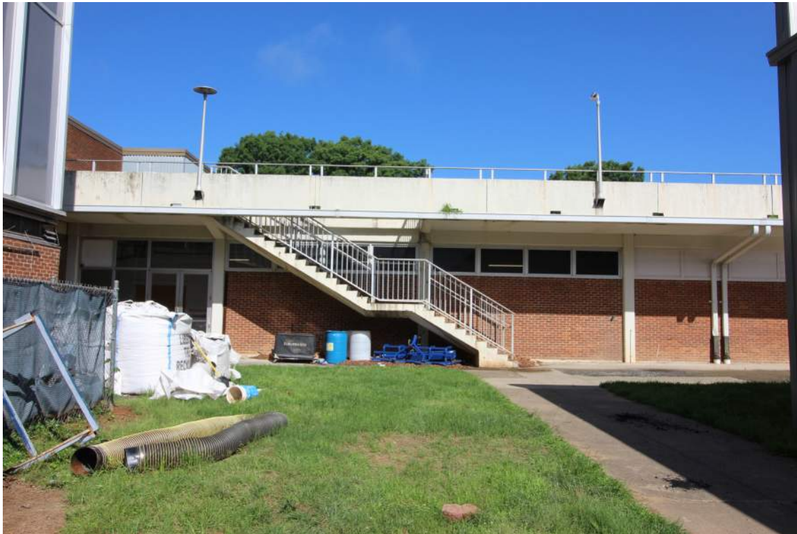
DHR Identification Number: 104-5292 June 4, 2018 Quinn Evans Architects Link, east elevation, looking west.
