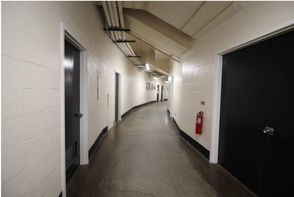
DHR Identification Number: 104-5292 June 4, 2018 Quinn Evans Architects 161 player level corridor, looking north.
